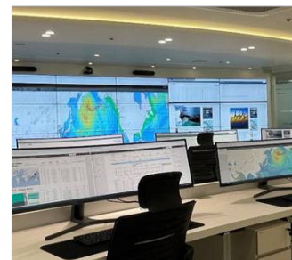
e-Center Control Room
